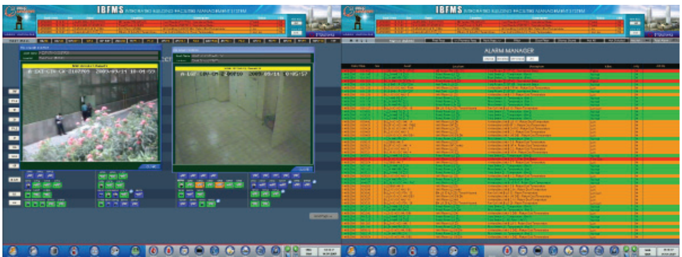
Figure 1.2 CCTV and Alarm Management - Users can view live CCTV integrated with Instek Digital's Alarm and DVR monitoring with their IBFMS software. Users can also see the cameras and hDVR statuses and locations.
